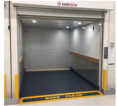
Freight Hoist entrance
