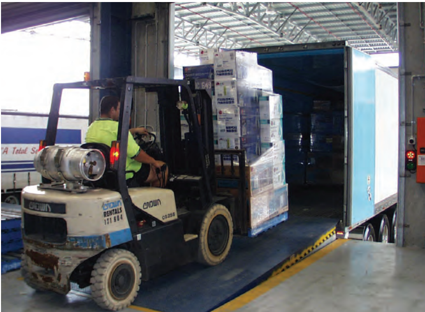
Typical model 710 Dock Leveller in action, safely bridging the height variance between trucks and loading dock floors
