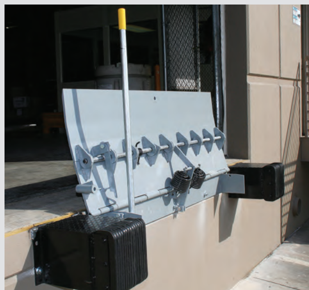
Mechanical Edge of Dock
