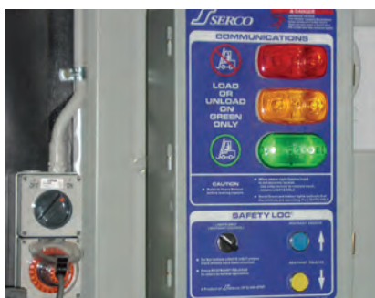
Pit Bull – internal LED Light Communication package and controls
