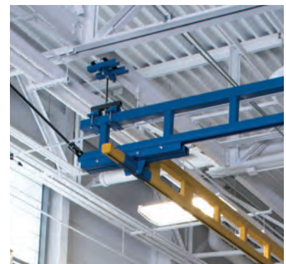
Ceiling mounted installations include brace to avoid any crane structural movement
