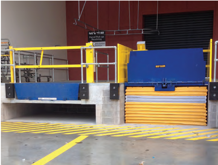
Retail Dock Installation includes gates for increased safety
