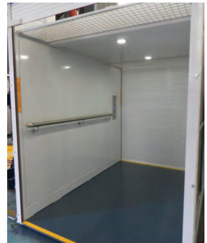
Freight Hoist with personnel hand rail
