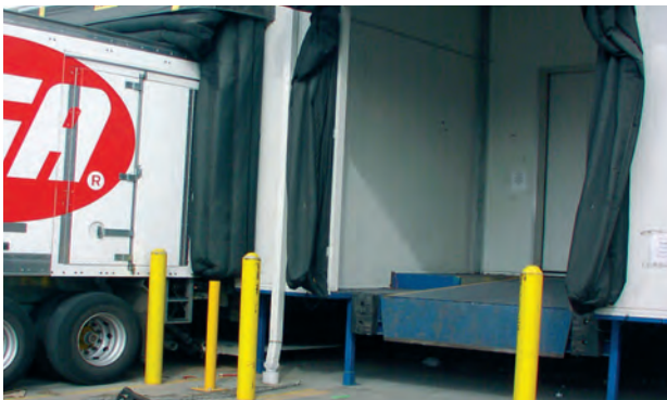
Stepped Down Igloo Dock Leveller application with inflatable dock shelters, maintaining the cold chain
